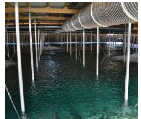
Filled More Ave. reservoir with in-tank aeration system in operation.
